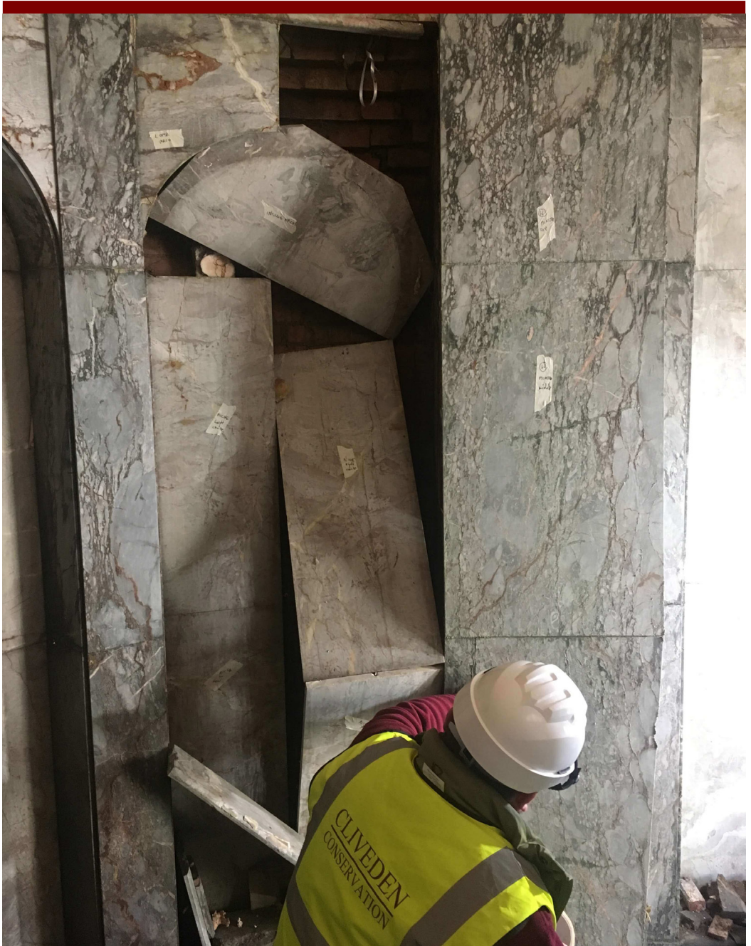
The marble cladding on the walls had fallen away dramatically.
